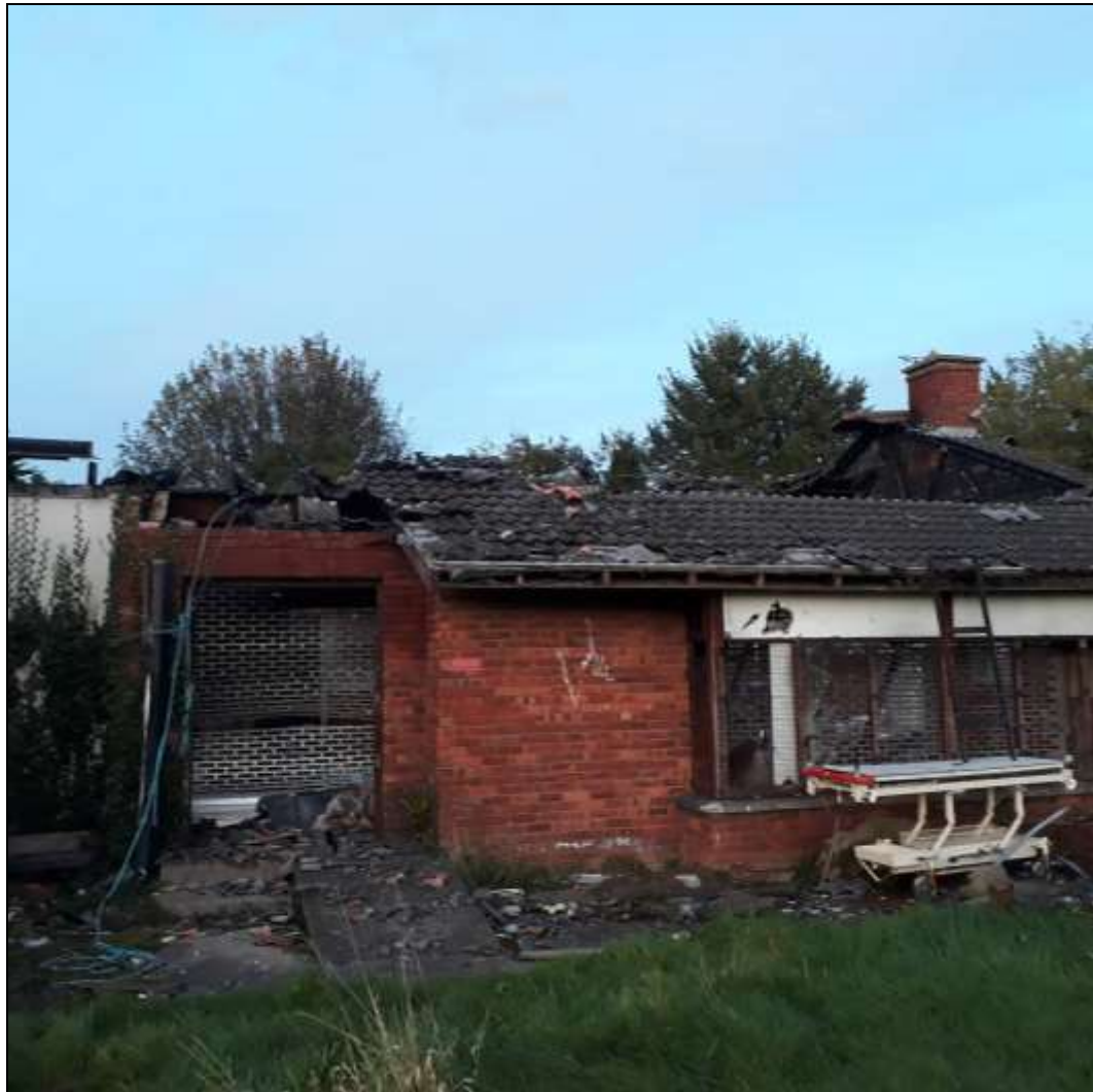
Plate 32. Rugby club building destroyed by arson.
