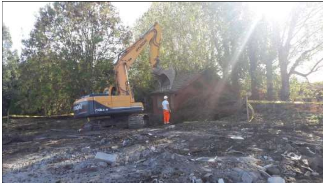
Plate 31. Roof stripping of the granny flat in the grounds of the easternmost house in October 2018.
